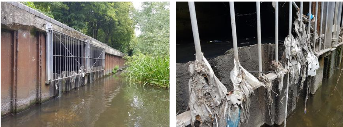
Figure 12 - Sewage rag caught on River Colne outfall in Watford
