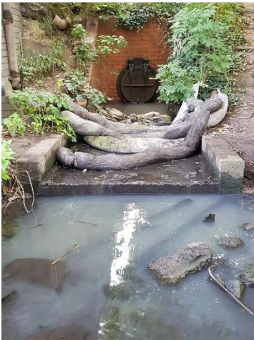
Figure 10 - Polluting outfall in Watford. Discoloured water flows from the outfall. Sewage rag and litter collects behind temporary blocks installed by Thames Water.
